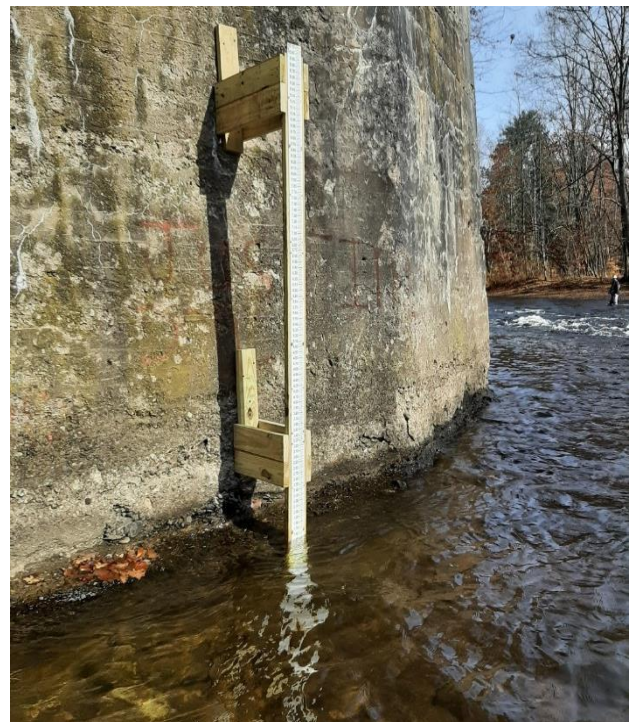
Figure 1. Staff gage installed on the north abutment at the Trestle Pool.
